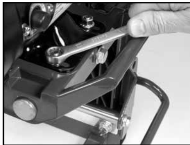
(E) Verify all motor mounting Bolts are tight
